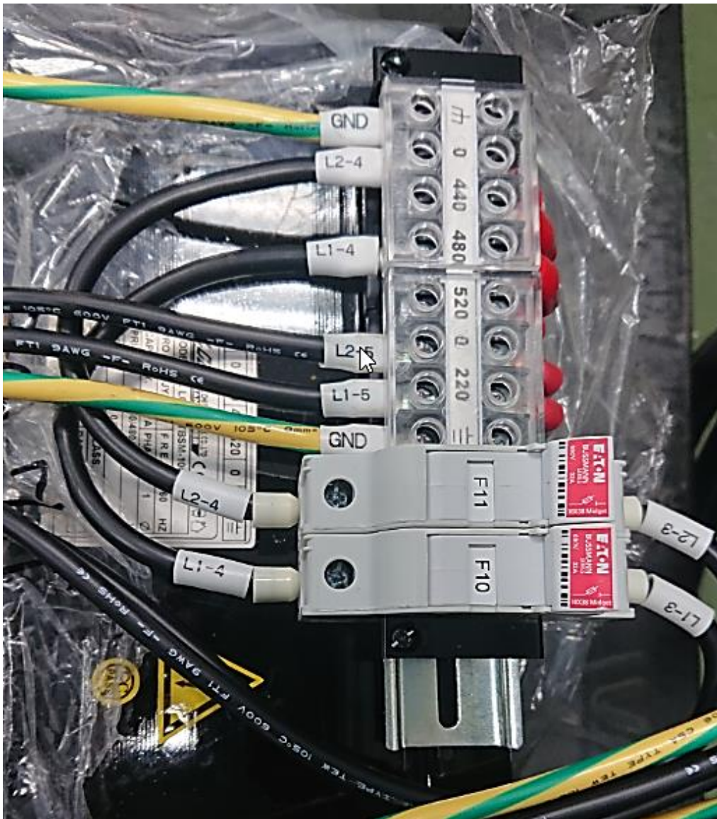
Figure 2.8.1 - Transformer Used on 480 Volt Machines
