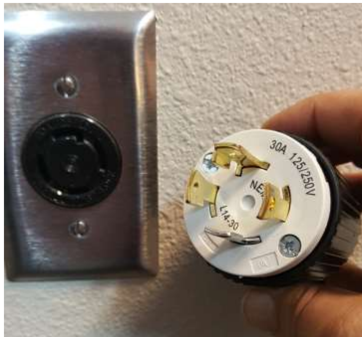
Figure 8.2.3 220 VAC Single Phase Plug and Receptacle
