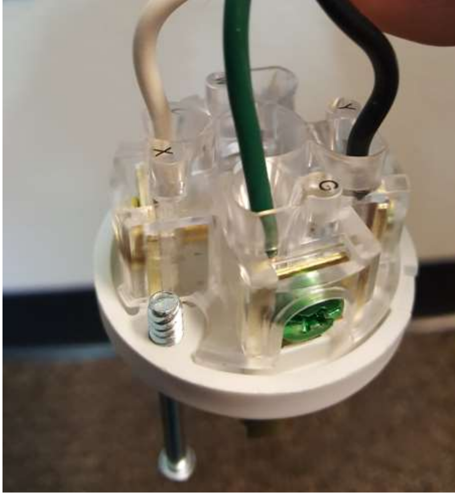
Figure 8.4 220 VAC Power Plug Wiring. Green = Ground. Black and White = 230 VAC single phase
